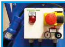
3-phase electrical panel
