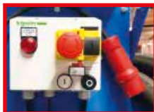
Single-phase electrical panel
